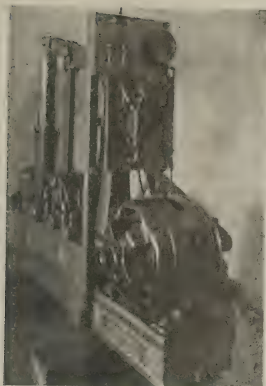
Motor-driven pumping unit
